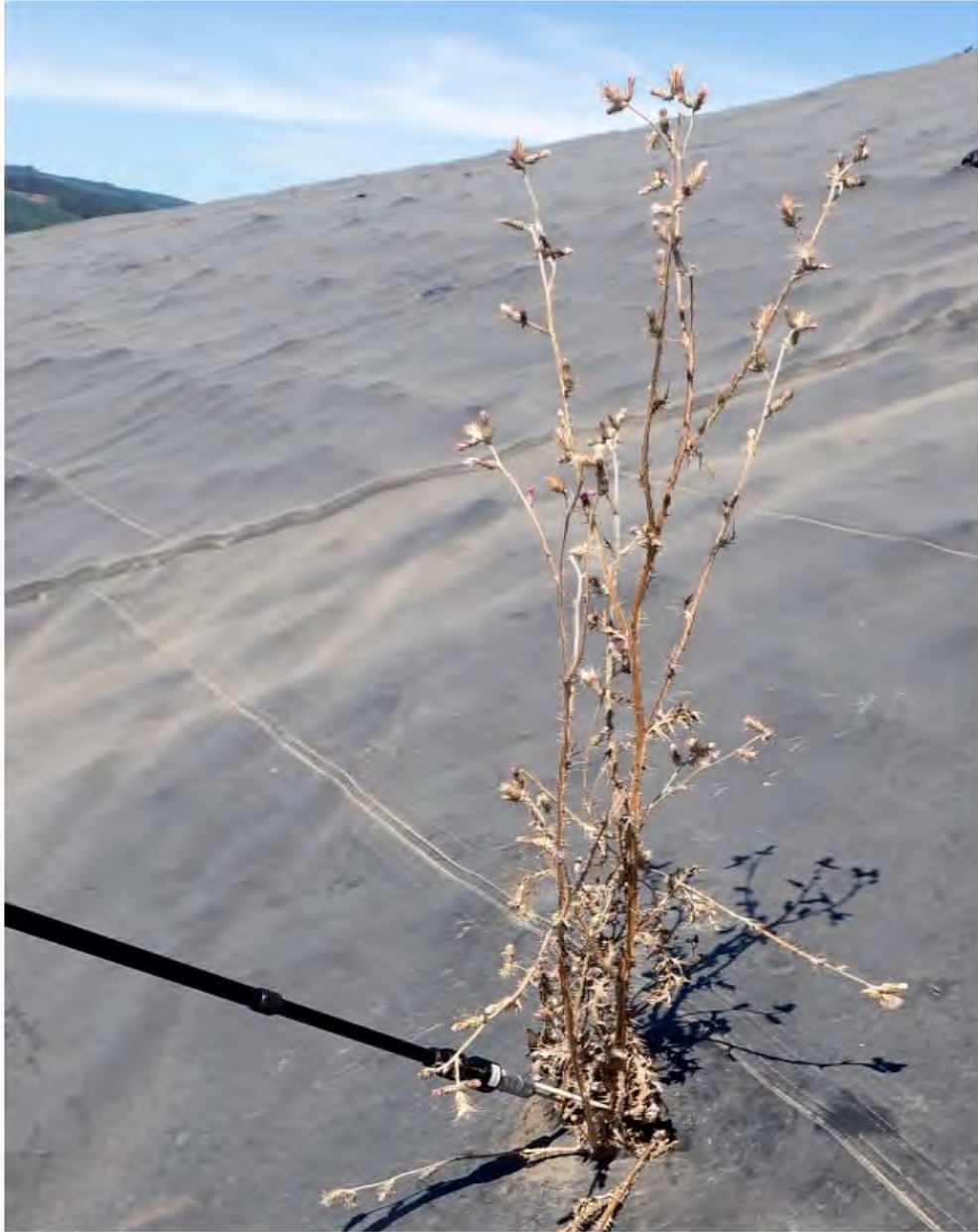
Example 3 - 800 ppm Methane Exceedance measured where a weed punctured the tarp
